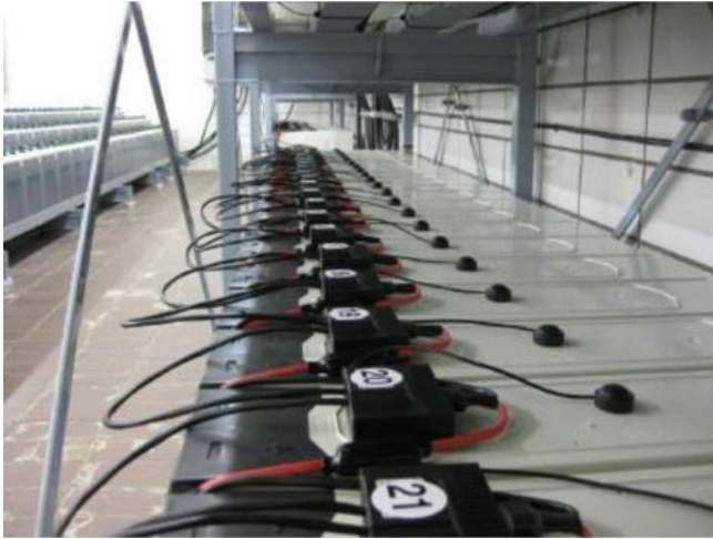
Civil Aviation Authority Installation, Europe
