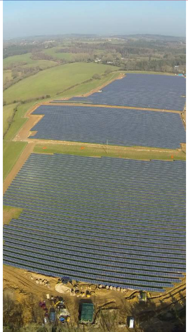
Solar farm constructed in Dorset, UK totalling near 7MW and 26,923 solar panels
