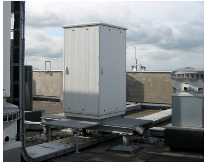
Roof mounted IP55 Outdoor UPS Cabinet
