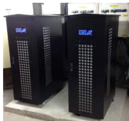
2x 80kVA High Internal Protection IP42 UPS supporting residential lifts in the UK
